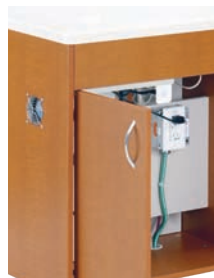
CPU module with Duplex electrical outlet and cooling fan
